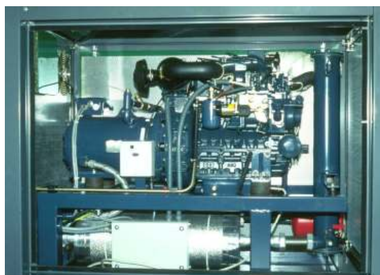
Figure 1: Rapeseed oil fuelled CHP-Unit 1
