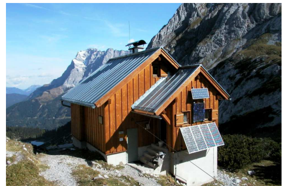
Figure 5: Housing of CHP with vegetable oil compatible combustion engine at "Coburger Hütte" in the Alps at 1920 m above sea level (picture: TFZ)
